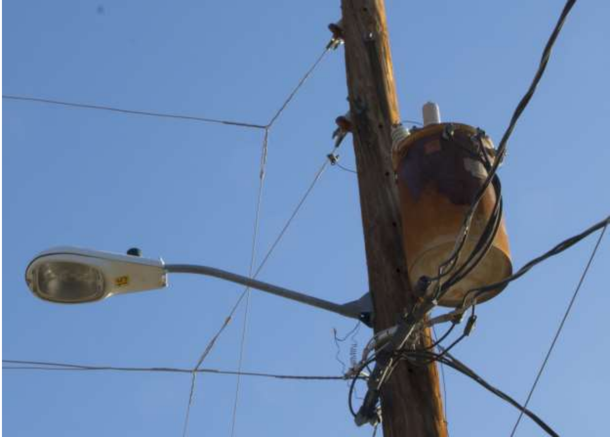
Figure 2.1 An operating distribution transformer showing visual indications of possible degradation.
